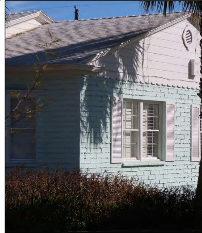
Image 19: Example of weeping mortar.
