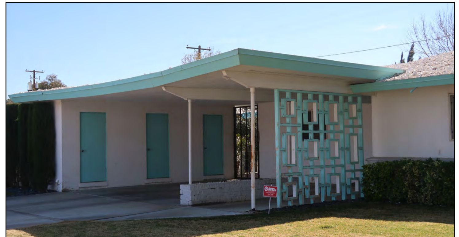
Image 12: Recommend retaining character defining features, including swooping roofline of carport and original wood screen.
