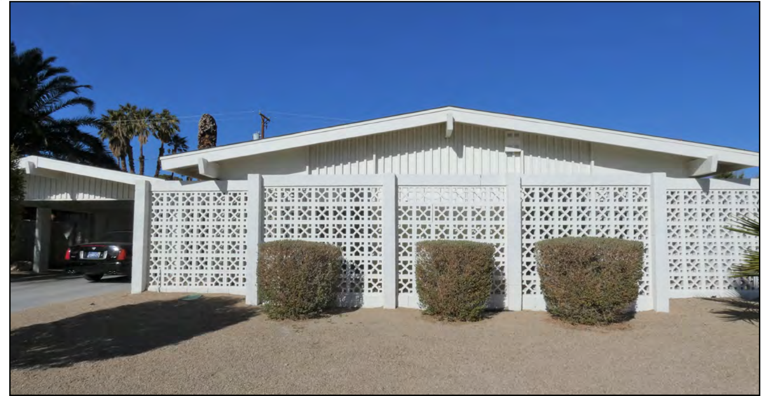
Image 2: Recommended enclosure that is compatible and reversible without removing or altering character-defining features.
